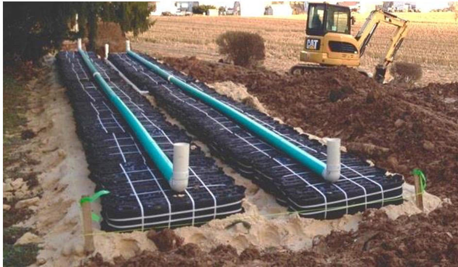
A 4-inch perforated distribution pipe is installed on top of the Eljen B43 modules.
