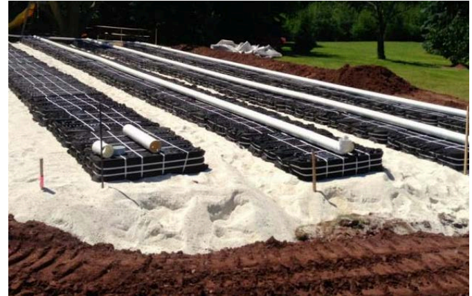
Four rows of modules are being placed on specified sand during the construction of this particular absorption area.
