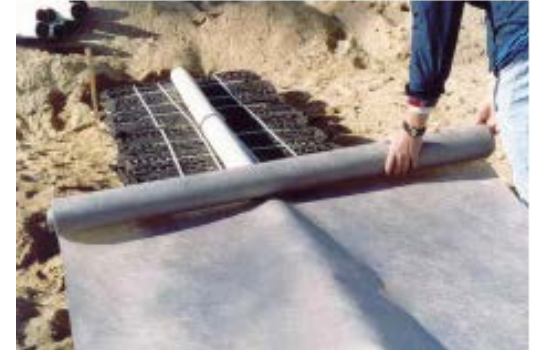
The cover fabric provided by the manufacturer is laid over the distribution pipe and modules.
