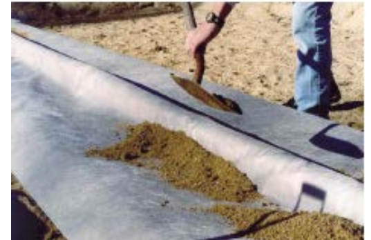
Specified sand is placed along the sides of the perforated pipe and over the modules.
